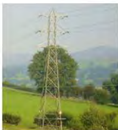
Steel pylons approx. 26m
